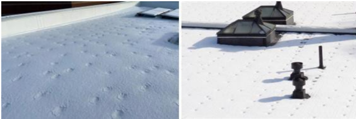
Figure 1. - Examples of thermal bridging at fasteners on snow-covered roofs.
